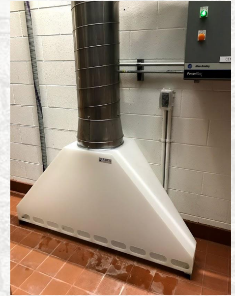
Cellar Extraction Ventilation
